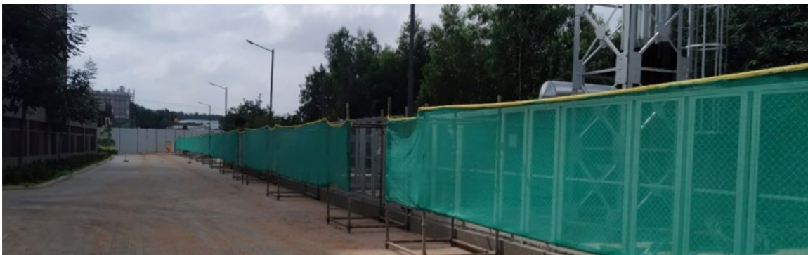
Pedestrian access with green shadow net provided for Tower D access
