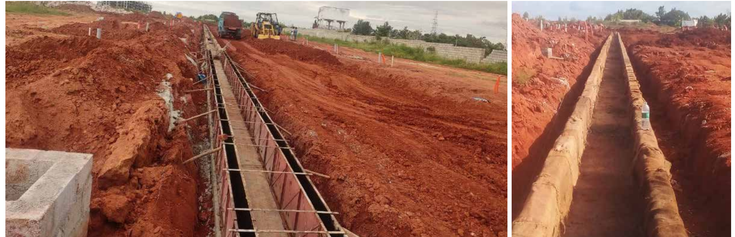
Storm Water Drain – Phase 1
