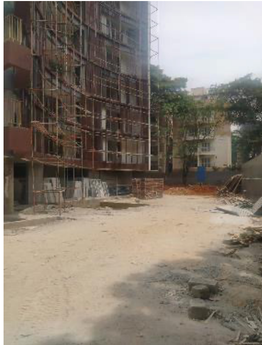
The external driveway and hardscape works for East, West & South Elevation are in progress.
