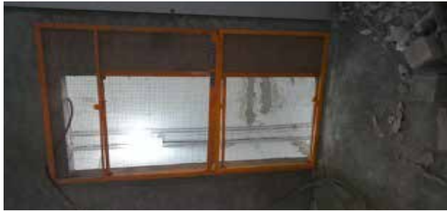
Barrication for lift openings
